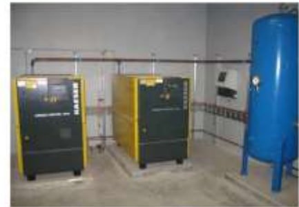
Two unit running (Base and trim)
